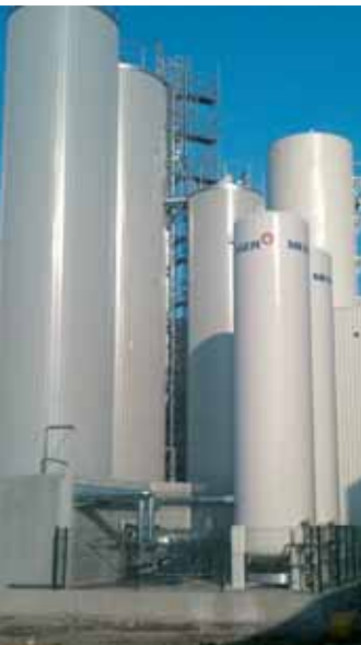
On-site-Anlage Thonon, 2010 On-site unit in Thonon, 2010
